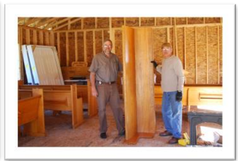
Fellowship member, Clay, from Arizona helped to cut down old, long pews so that they could fit in the chapel.
