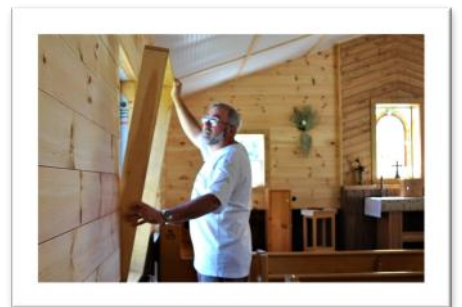
Fr. Alan works on building and installing all the interior window boxes and trim.
