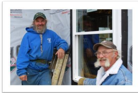
Dear friends and neighbors, Lloyd (we call him Pilly) and Ron, graciously helped to install our windows.
