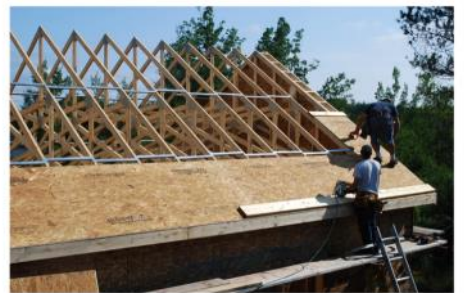
Sheathing and shingling the roof. What a wonderful day to finally stand in the chapel with a roof over our heads!
