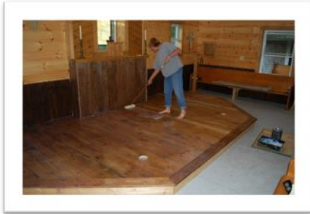
Sue applies several coats of floor-grade polyurethane to the platform. The rest of the floor will hopefully be installed next summer.
