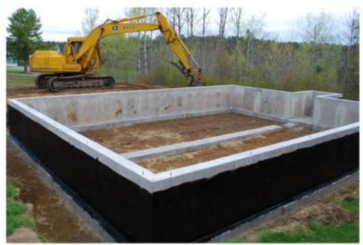
With the excavation and foundation work complete, it's time to backfill up to the frost wall and begin the subflooring.
