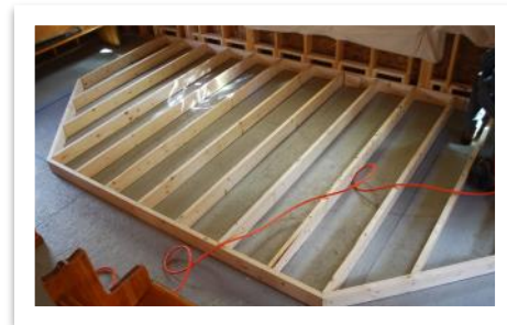
Fr. Alan and Sue build the framework for a raised platform in the front of the chapel.
