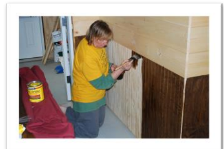
Sue works on staining the wainscot that wraps around the whole interior of the chapel.
