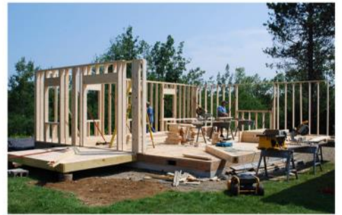
It was an amazing process as we watched local carpenter, Terry, frame up the walls. What a thrill as we witnessed the chapel taking shape.
