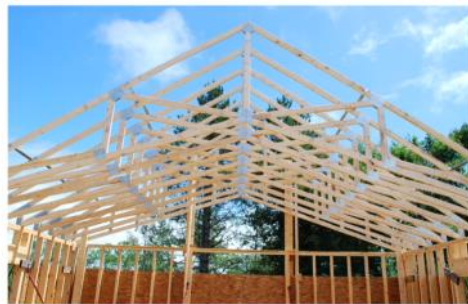
One by one the roof trusses were raised and fixed into position.
