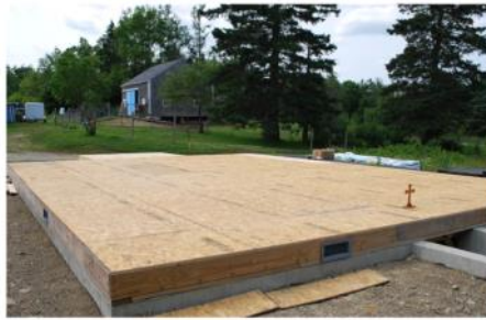
With subflooring complete, a cross is set up to mark the location of the future altar.
