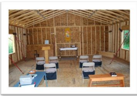
Even without lights, heat, or windows, we moved the services into the chapel during the summer months.
