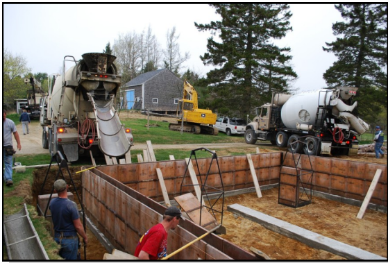
FRONT LEFT: Groundbreaking for Holy Trinity Chapel began on Monday afternoon, 5-6-13. FRONT RIGHT: Our general contractor, Terry Stevens, makes quick work of the site preparation. TOP LEFT: The foundation crew begins to lay out the forms for the footers. TOP CENTER: A young visitor, Thomas Gardner, watches as cement is poured into the forms. TOP RIGHT: The crew from Richardson & Son keeps the cement moving along. MIDDLE LEFT: Later that same day the molds are set in place for pouring the frost wall. MIDDLE CENTER: This morning (Ascension Day) at 6:30 AM the cement truck returns to begin pouring the walls. BOTTOM LEFT: By 8:00 AM a second truck comes to help finish the pour. BOTTOM RIGHT: By 10:00 AM the walls are poured and the crew is finished!
